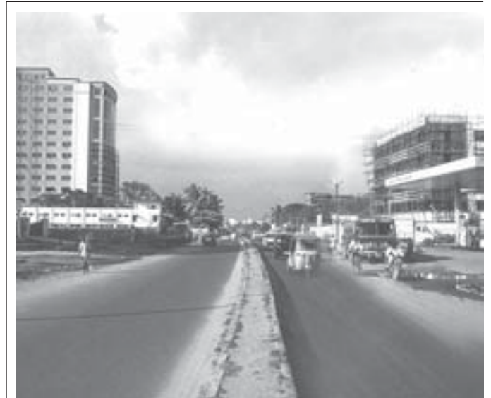
Work gets underway on the IT Highway in Chennai. (Picture by V. RAJESH.)
