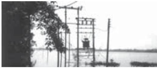
With floods come the danger of electrocution as the rising waters come into contact with live wires. Illegal tapping into the grid by many Indians who cannot afford to buy electricity adds to the potential hazard. Photograph: Donovan Wyle.
